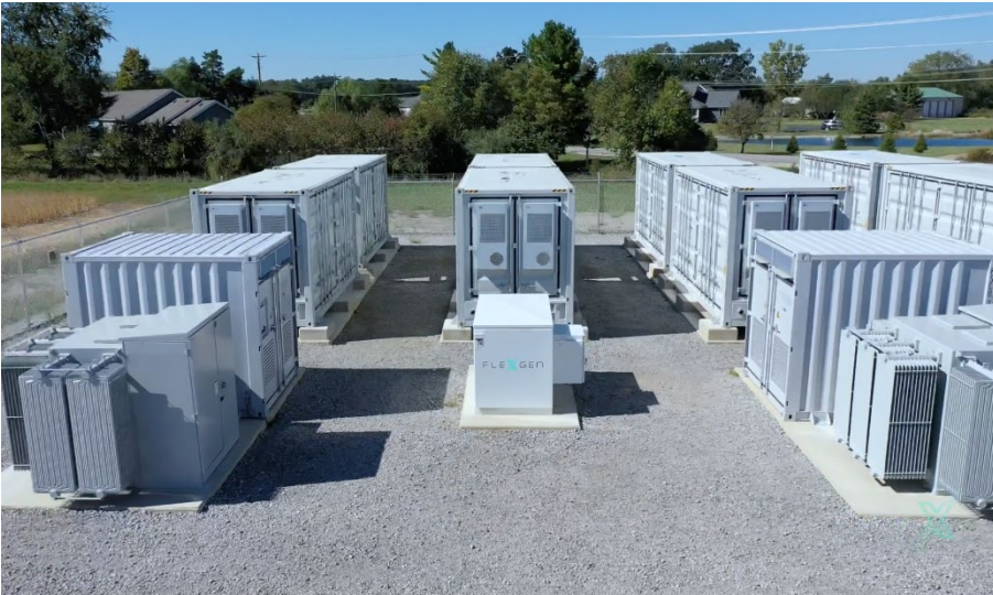
Operational 18 MWh facility, Indiana
