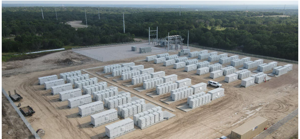
Operational 100 MWh facility, Texas
