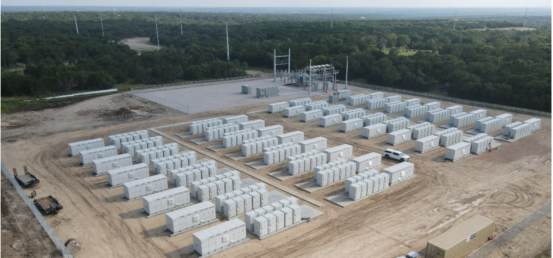
Operational 100 MWh facility, Texas
